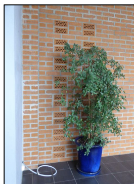
Alt. tilluft via hull i teglstein
